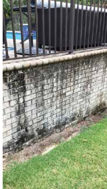
dirt, stains and mold growth, diminishing their appeal and safe-
