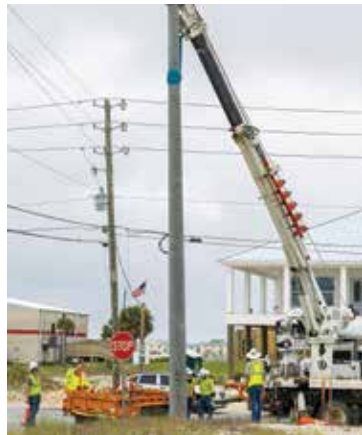
Crews install a concrete power pole in Northwest Florida to improve resiliency during hurricanes and severe weather and also enhance reliability during day-to-day conditions.
